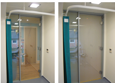
LC SmartGlass Doors – Treatment Room Entrance
